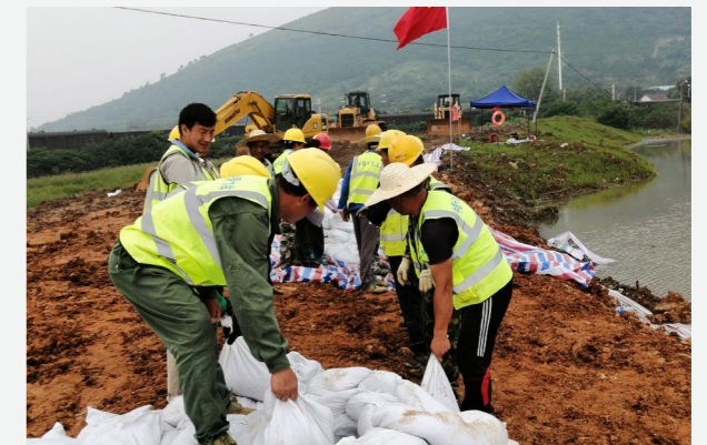
Employees of MCC19 made every effort to fight floods and protect production in Chaohu East Outer Ring Project
